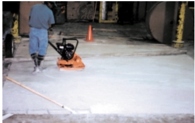
Re-grading and leveling the surface is an important first step before laying any decorative floor system.
