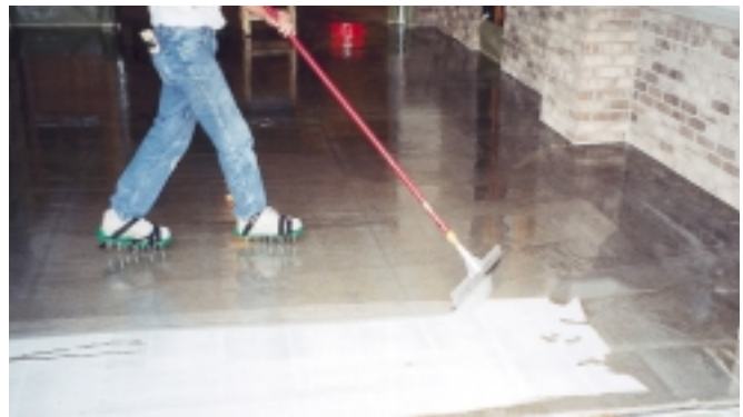
Before this man could squeegee and backroll a mixed epoxy basecoat, the surface prep team had to employ a shot-blast machine to remove laitance and unsound concrete created by excessive power-troweling during the cement pour. Note the use of spiked shoes that allow the crewman to walk on the wet basecoat. The spike marks will level themselves out.
