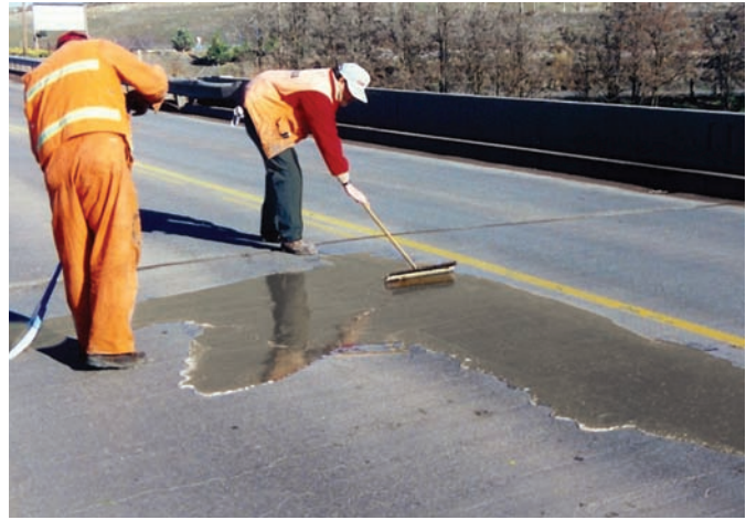
The Contractor spreads the epoxy over the deck surface with a broom or squeegee and directs the material into all open voids.
