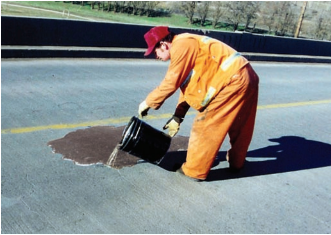
On smooth surfaces, the mixture can be poured directly onto the cleaned concrete surface, covering the cracks.
