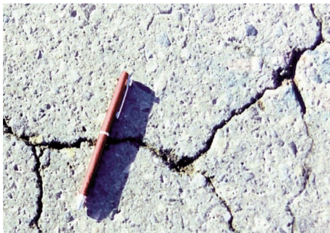
Close-up of cleaned concrete deck and trapped dust and debris in the cracks before being blown out clean with air.
